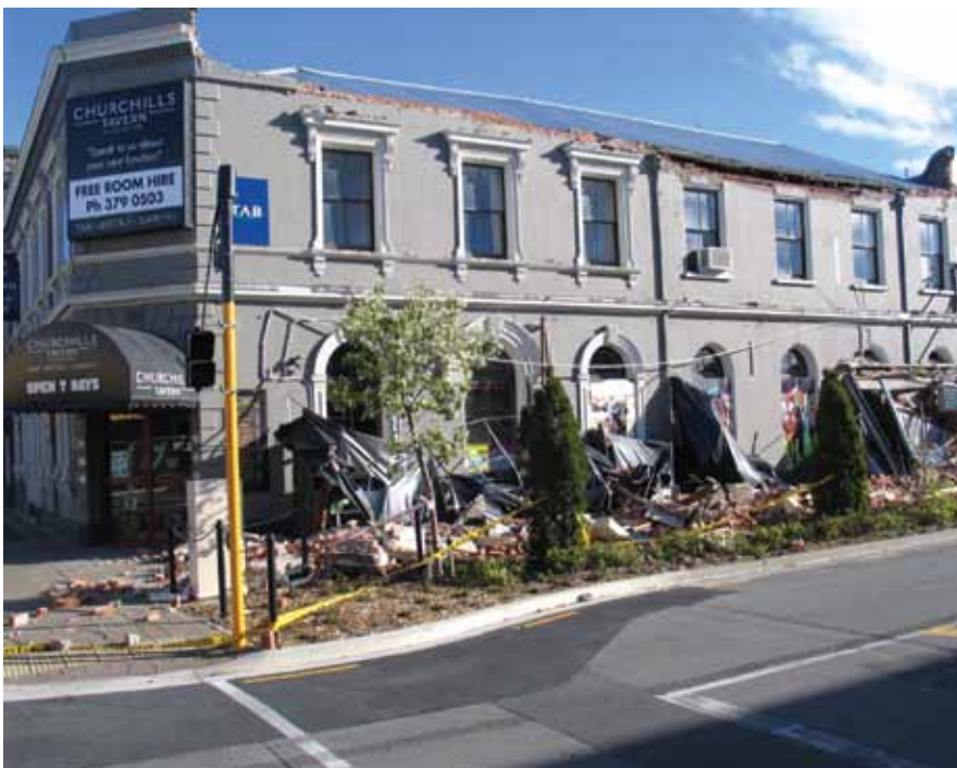
Figure 3. A portion of this unreinforced masonry wall in Christchurch, New Zealand fell onto an outdoor café. Fortunately, no one was there. The U. S. has many buildings like this.
