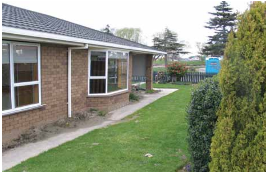
Figure 4. Subtle but expensive damage from liquefaction in Christchurch, New Zealand. The house, relatively undamaged, has settled about eight inches, which will cause storm drainage from the entire lot to run to the house. Regrading the lot is not always an option due to the adjacent street elevations.
