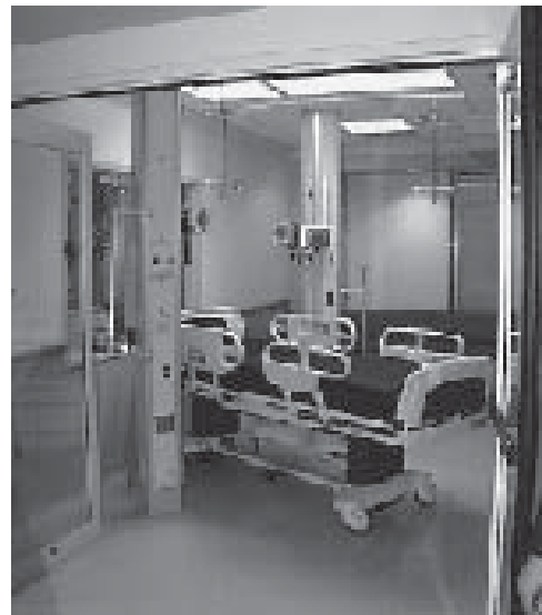
Twin power columns MICU, Methodist, Houston.
