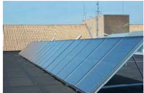
Figure 7 At Aabenraa hospital three solar collector systems were implemented. All the systems were roof mounted. For architectural reasons and in order to avoid glare, solar collectors were mounted so that they aren't visible from outside the building. Special attention was given to the risk of legionella bacteria, by using electrical backup system to ensure that high water temperatures required for avoiding legionella growth were always achieved. Each system includes approximately 50 m 2 solar collectors, which provides an annual energy yield of about 27 MWh per system. This provides about 60% of the annual energy requirement for water heating.
