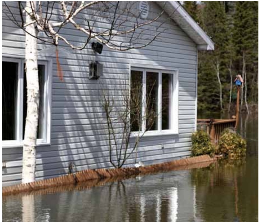
Snow that melted too fast caused this home to flood in 2008.
