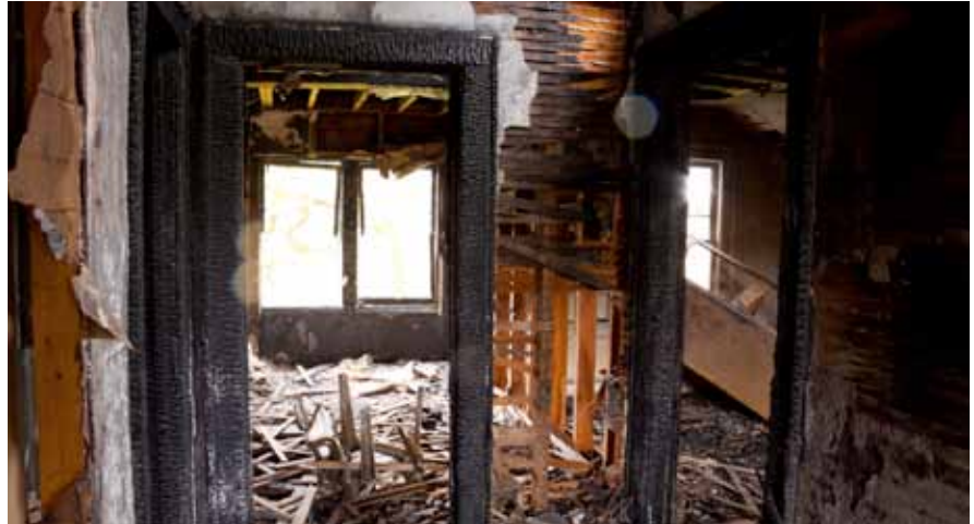
Firefighters couldn't stop the flames that swept through this family home.
