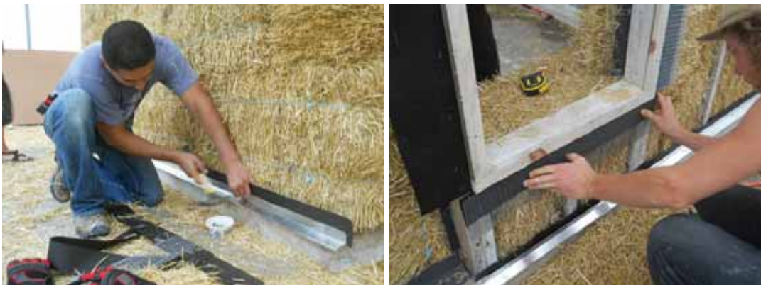
Figure 2: Application of air-fins, flashing, and metal lath at critical transitory locations along the wall plane.
