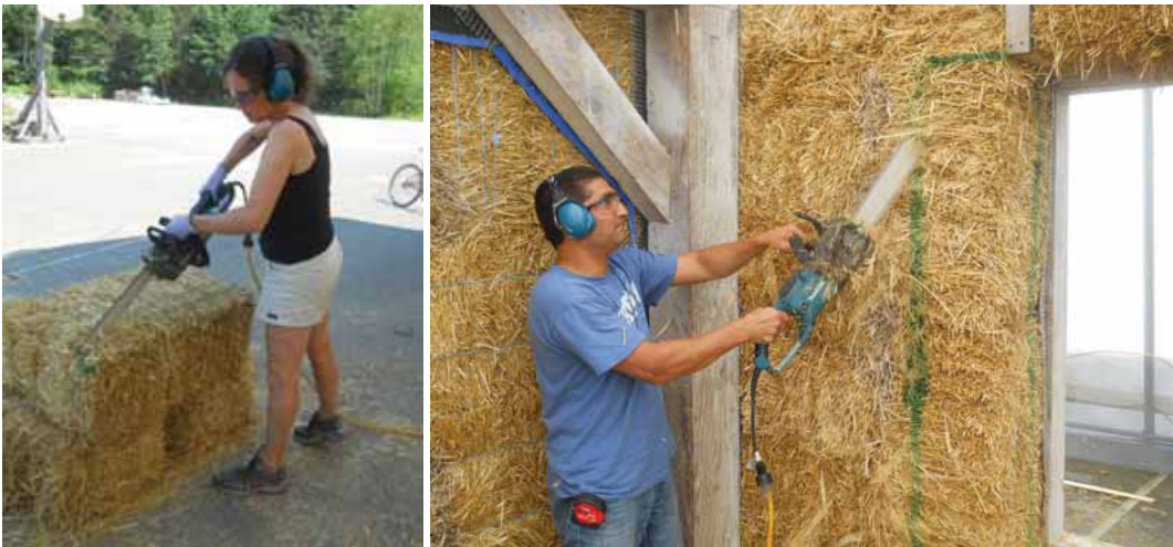
Figure 1: Squaring of bales (prior to installation) and beveling of window wall edges with chain saw.
