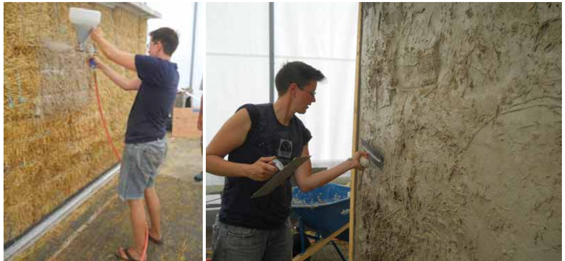
Figure 3: Spraying clay slip (drywall texture gun and air compressor) and two-hand trowel plaster method.
