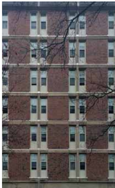
Figure 2: Thermal bridges with exposed concrete.
