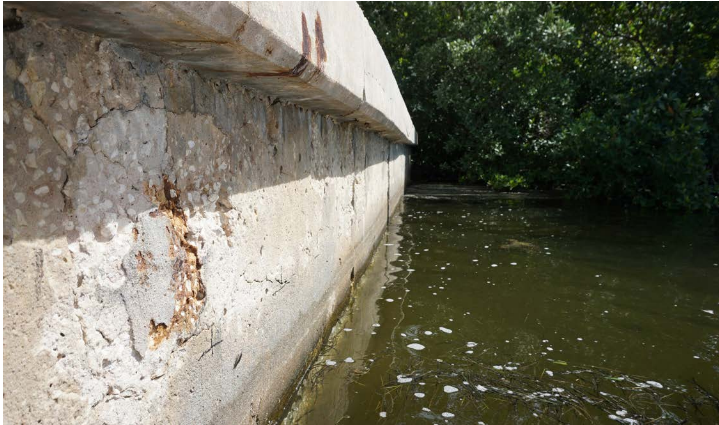
Figure 11. Aging seawall near Englewood, FL. Over time, seawater weakens cement and infiltrates the wall, causing rebar to corrode.
