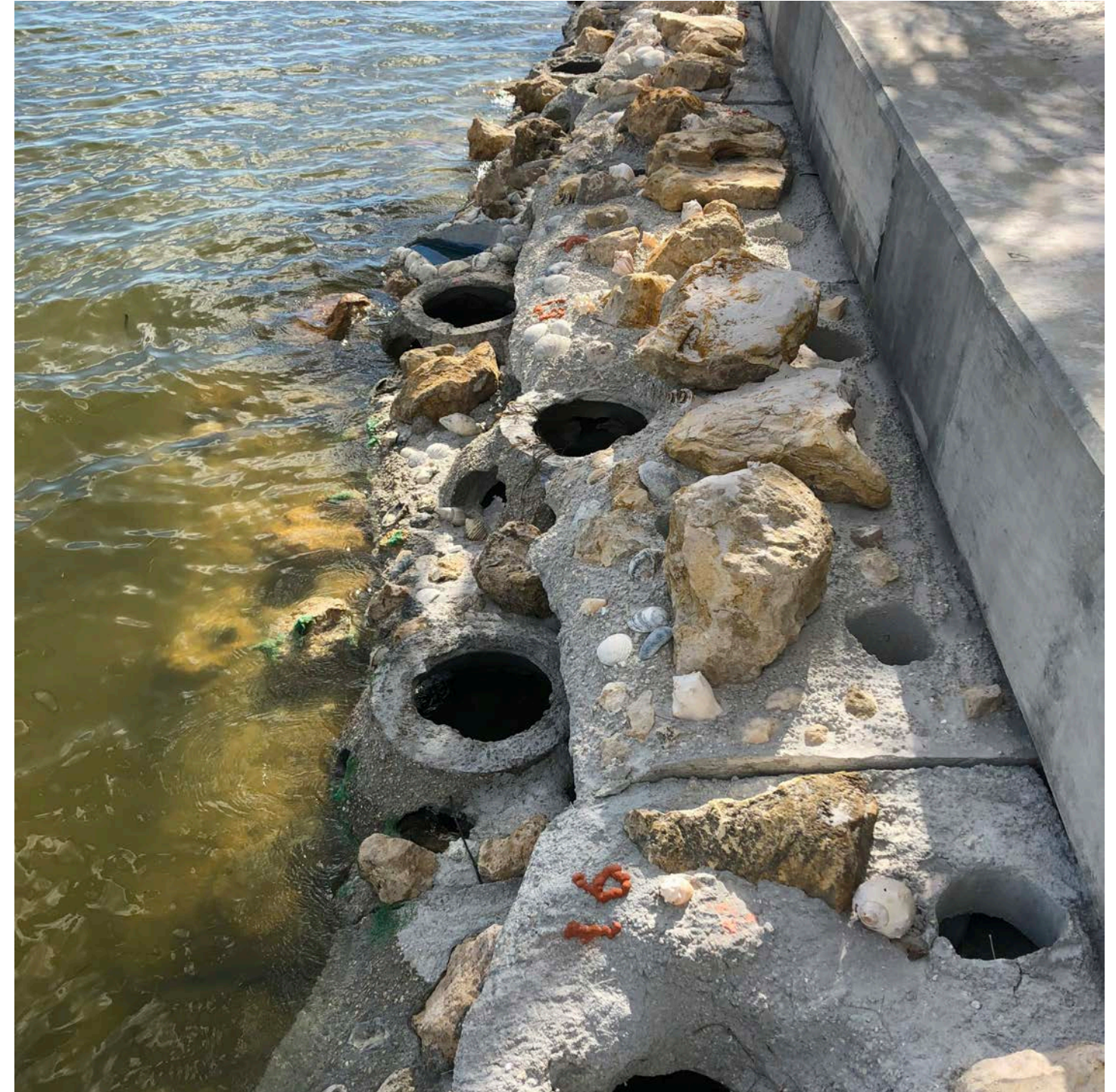
Figure 15. Reef Balls were integrated into a stepped concrete living shoreline installed in Sarasota. Production of the modules involves embedding Reef Balls into slabs of concrete poured over layers of sand to create levels.
