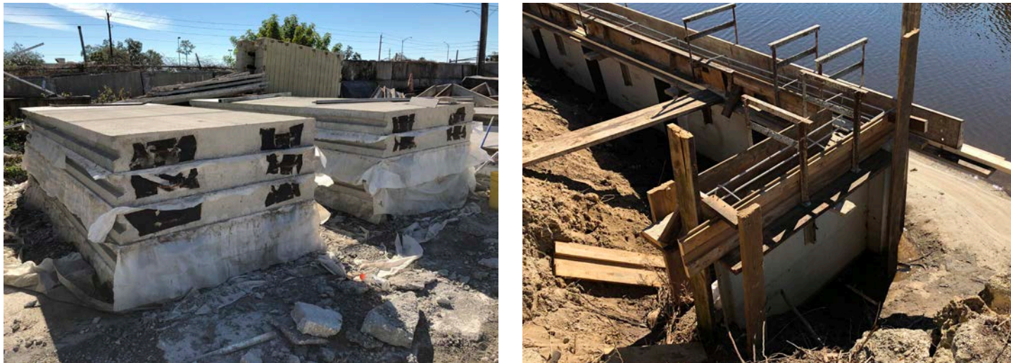
Figure 12. Installed as precast panels with a cast in place cap, concrete seawalls are the most widely used panel type historically. The harsh transition from water to wall precludes any tidal zone for species.
