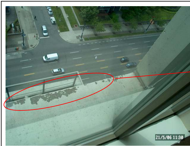
PHOTOGRAPH 2: View of the outward projection of a floor slab from the interior of the building. Note the spalling paint on the surface of the slab.
