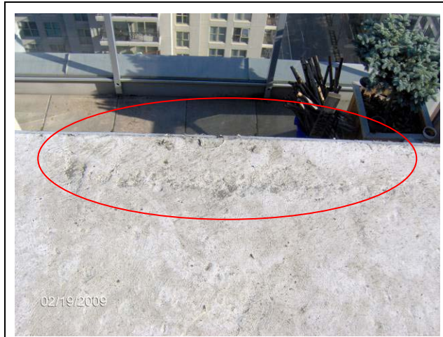
PHOTOGRAPH 5: The ellipse denotes an area where the silicone paint has delaminated from the concrete slab.
