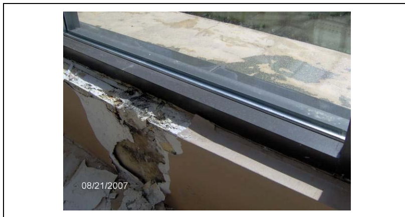
PHOTOGRAPH 10: Shows the consequence of utilizing a storefront window system in a location exposed to wind-driven rain without adequate sub-sill waterproofing. The sub-sill flashing in this photograph had a joint at the point of the leak.
