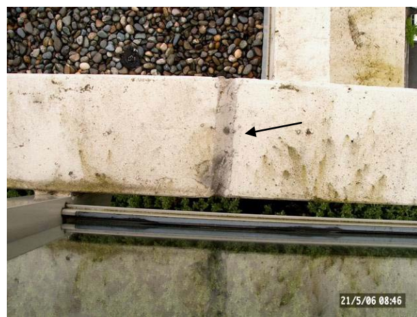
PHOTOGRAPH 7: The top of this parapet wall, on a building located approximately 10 blocks away from the building shown on Photograph 5. In this case, a joint in the parapet wall is waterproofed with sealant, thus increasing the likelihood of leakage.
