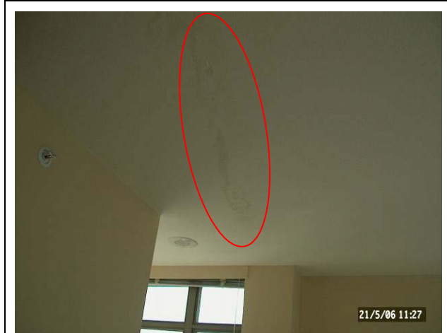
PHOTOGRAPH 4: The ellipse denotes a crack in the ceiling where water was dripping.
