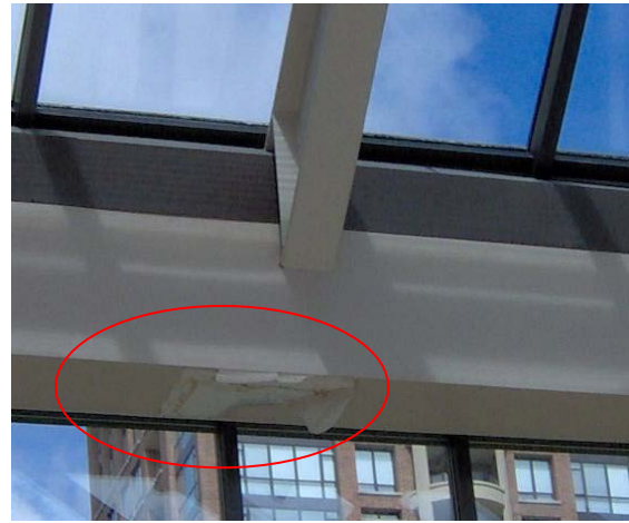
PHOTOGRAPH 13: Damage to the ceiling caused by the leaking of a very large skylight without the raised leg overlapped drainage gutters.
