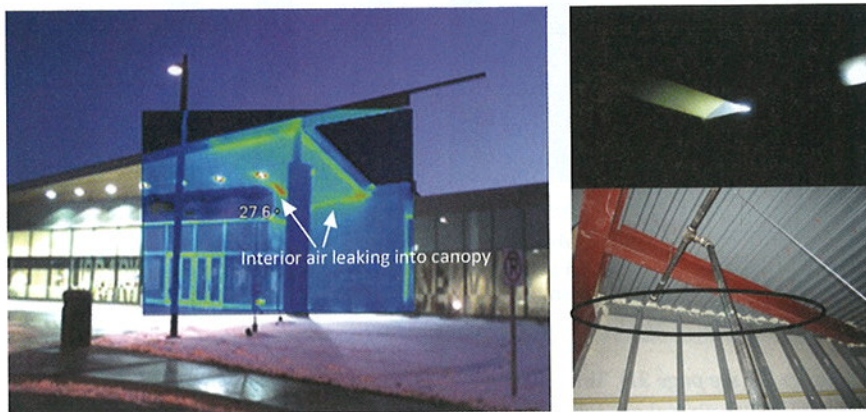
Figure 3: IR image of canopy air leakage (left), with gaps circled (right) between the wall and the corrugated roof deck.
