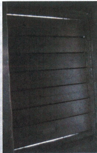
Gaps at the top and bottom of an outside air damper.
