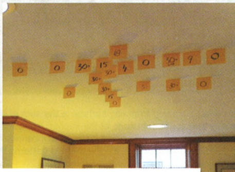
Figure 5: Ceiling moisture measurements.
