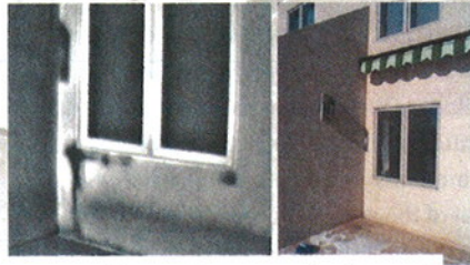
Figure 7: Three patterns—sun shadow and splash water, along with moisture, in EIFS.
