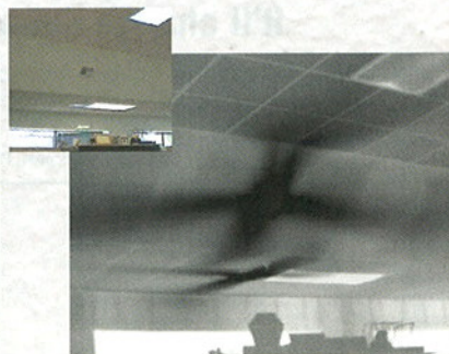
Figure 2: Supply air diffusers.
