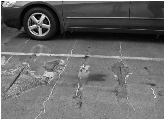
A Corrosion of embedded steel reinforcement is a leading cause of premature deterioration in parking garages.
