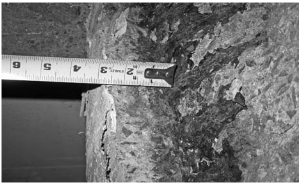
▲ Sufficient concrete cover over reinforcing is essential to protect embedded steel from water and dissolved chlorides.
