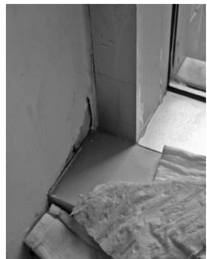
▲ New high-performance windows installed adjacent to conductive wall assemblies can still lead to condensation and moisture damage.
