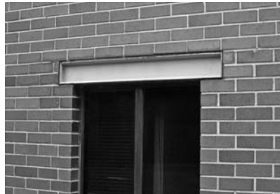
▲ This steel lintel acts as a thermal bridge, conducting heat through the building exterior.
