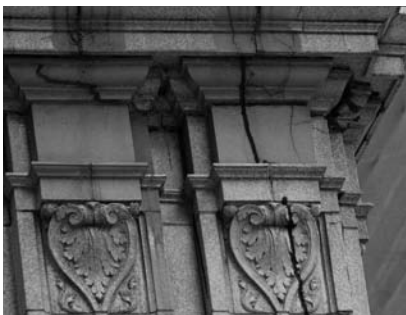
A Cracking at building corners.
