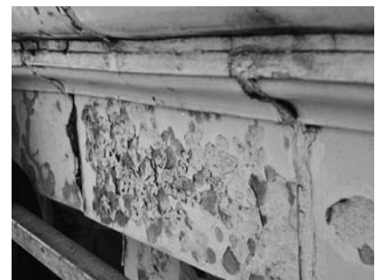
A Blistering coating.
