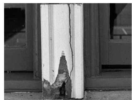
▲ Crack and spall caused by corroded steel.
