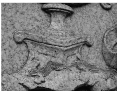
▲ Failed prior repair effort.
