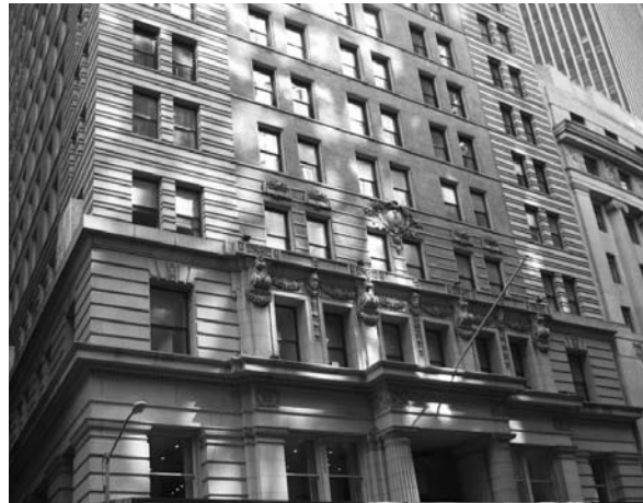
▲ Broad Exchange Building, 25 Broad Street in New York, New York. Landmark Terra Cotta Facade Restoration.
