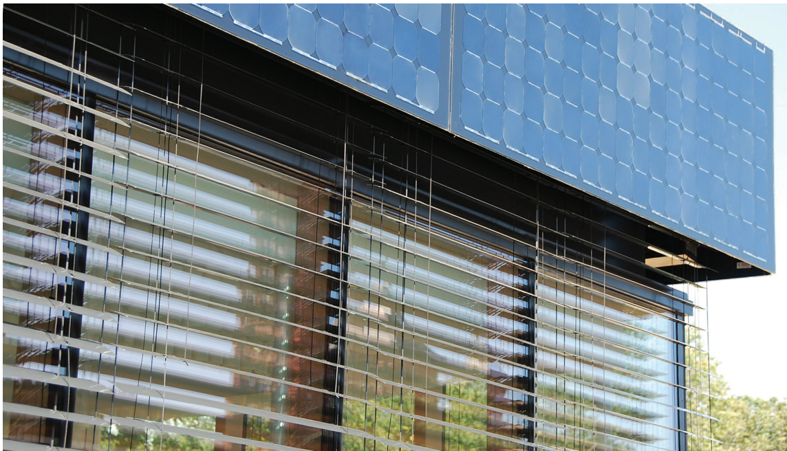
Figure 3: Detail of BIPV fascia at southeast corner with exterior shades open (Photo by Terri Boake).
