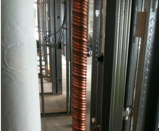
Figure 17: Copper pipe for shower drain heat recovery.
