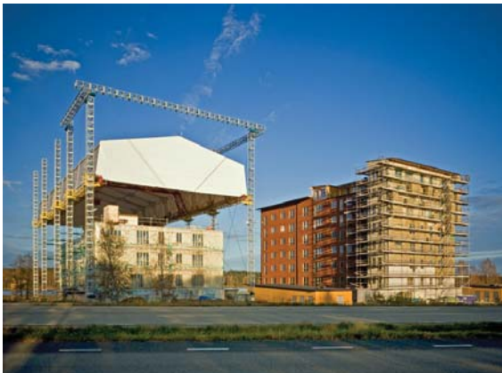
Figure 9: Limnologen's rising tent structure for weather protection during construction (Photo credit: Midroc Property Development).
