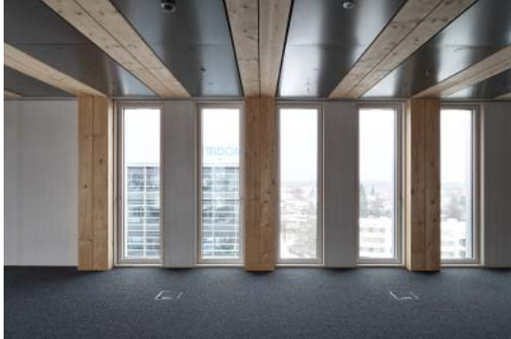
Figure 7: Ceiling panels between timber beams conceal systems at LCT ONE (Photo Credit: www.creebuildings.com).
