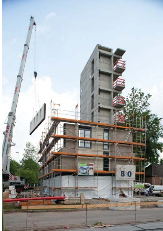
Figure 8: Holz8 building employed pre-cast concrete for the cores, contributing to a very quick construction time of 16 days (Architecture by: Schankula Architekten, Photo credit: Huber & Sohn).
