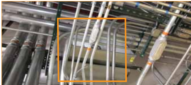
Figure 3. As highlighted in this box, the maze of conduit has blocked access to the relief fan.
