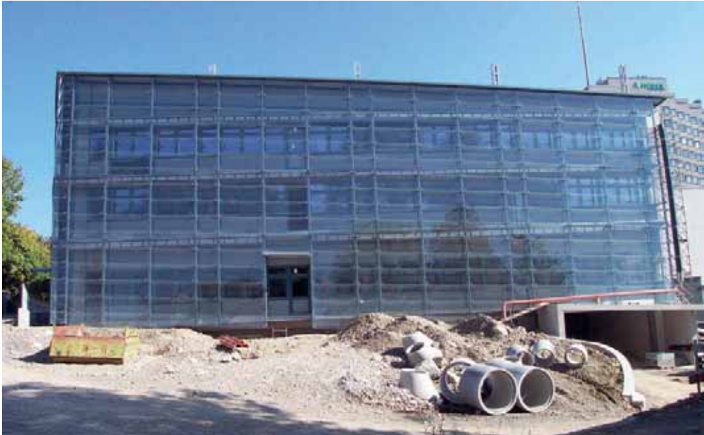
Figure 8 West façade showing double skin with operable windows behind an outer layer of glazing.
