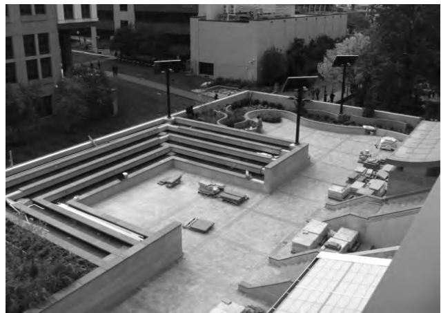
▲ After: Renovation provides varied program space that incorporates plantings, solar lighting, and durable materials.
