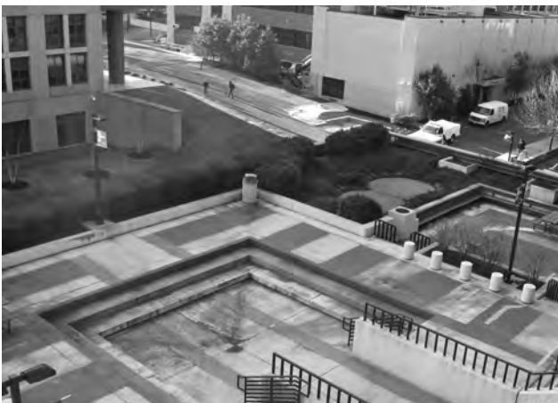
▲ Before: The under-used plaza at this public university showed signs of age and wear.
