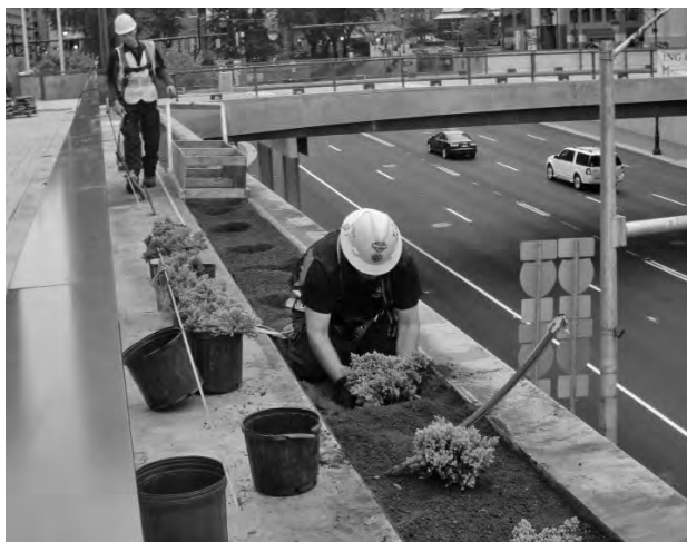
▲ Plan ahead for planter care and upkeep by installing linear fall protection lines for safety harness tie-ins.
