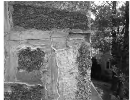
▲ Deteriorated face-pointed mortar.
