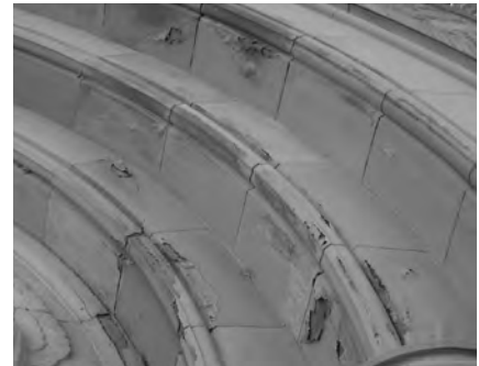
▲ Blistering waterproof coating.
