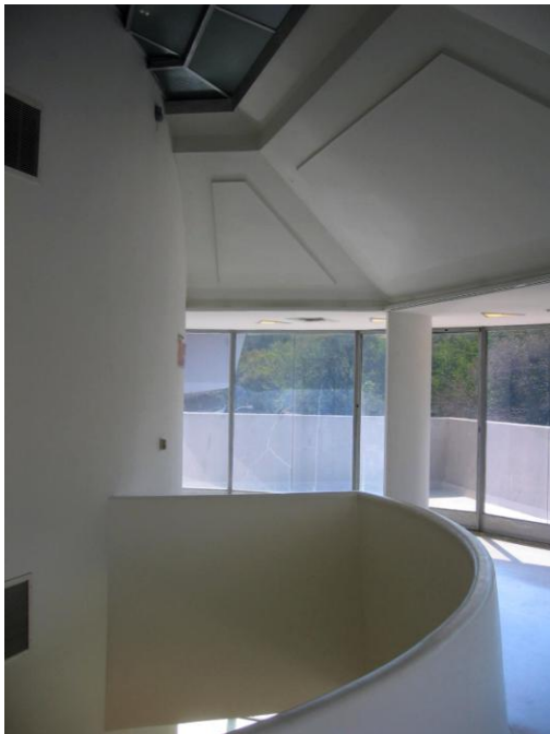
Fig. 3: Existing single-glazed steel-frame glazed enclosure at the Guggenheim Museum. (2005) © Angel Ayón, WASA/Studio A.
