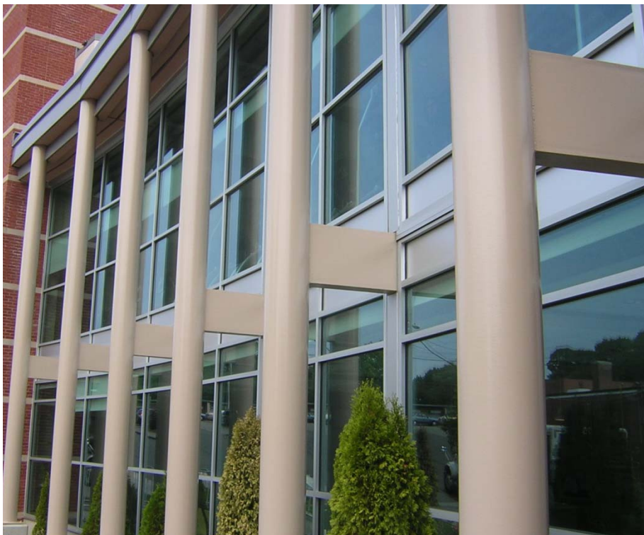
Figure 12 - These exterior steel columns are heat sinks, drawing heat from the beams that penetrate from the conditioned space. Beams inside the building were dripping wet.
