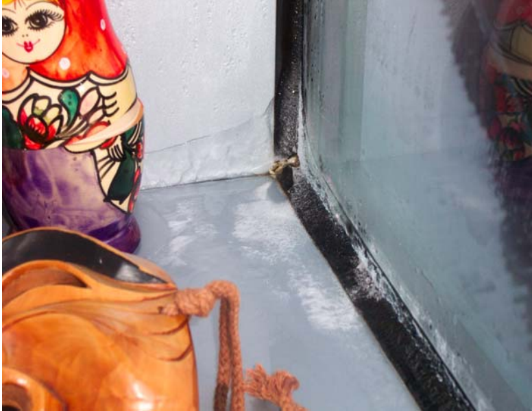
Figure7 - Frost on a curtain wall frame due to lack of primary air barrier seal.
