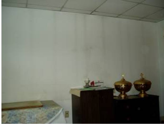
Figure 11 - Steel studs lowering temperature of interior surfaces causing ghosting
