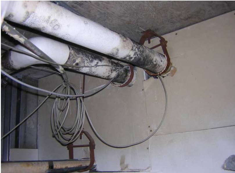
Figure 2 - Infiltrating warm humid air into this air conditioned plenum caused condensation on cold surfaces of chilled water pipe insulation.
