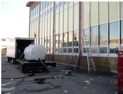
Figure 33: Portable water reservoir and pump system.
