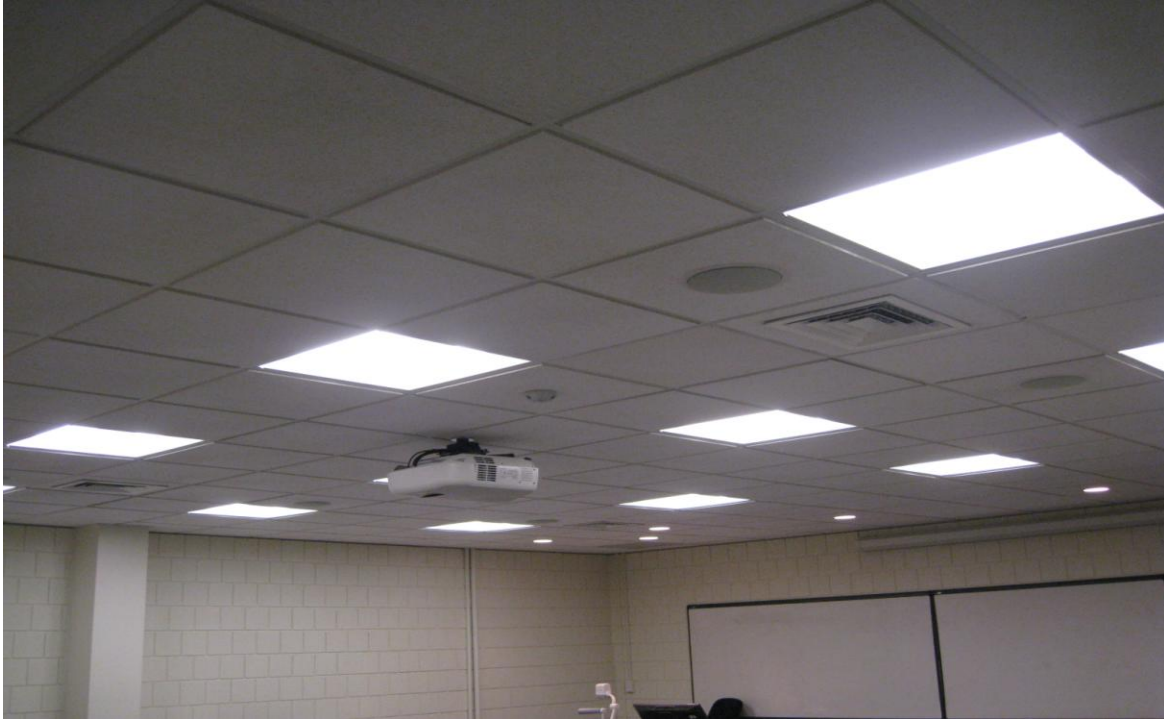
SMART CLASSROOM 124 CEILING WITH SPEAKERS AND AC DIFFUSERS
