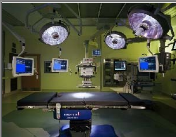
Photo courtesy of KMD Architects Green downlights reduce eye fatigue, improve visibility, and enhance the viewing of video images in the operating room.
