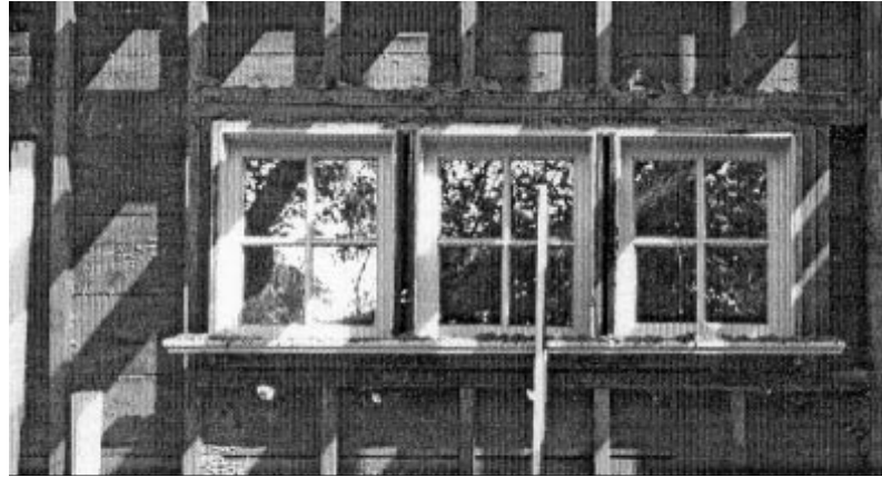
Figure 1: Walls of a wood-frame house built in 1919 at the University of Saskatchewan were retrofitted from the exterior with CFI in 1926 and opened in 1975. Inspection showed no traces of moisture and no visible damage.
