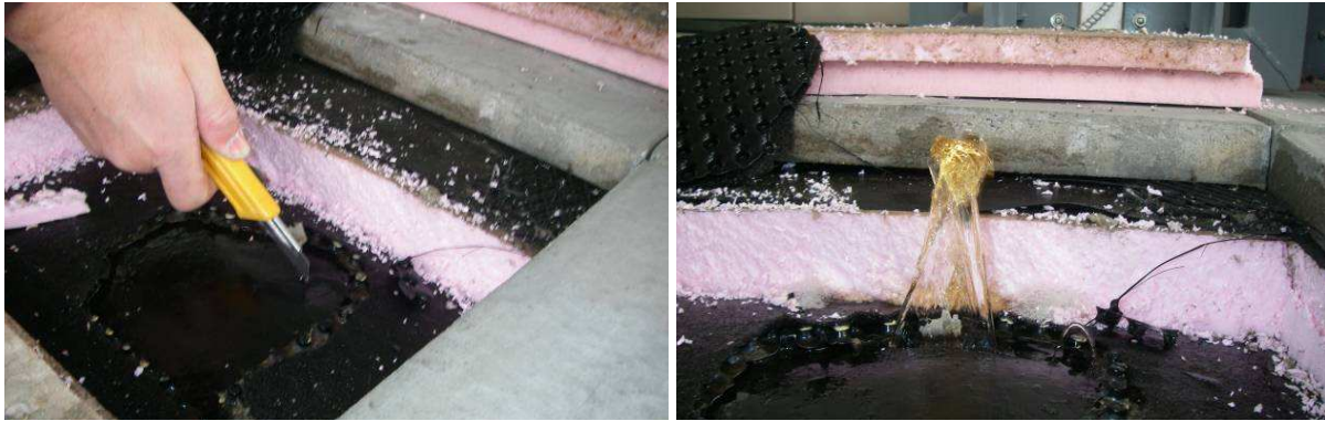
Figure 11 & Figure 12: Cutting of Membrane Blister and expulsion of water during extraction process.
