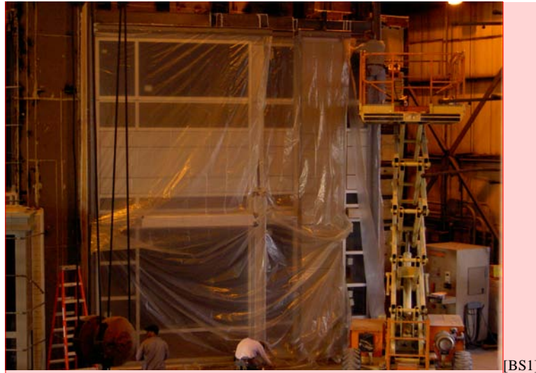
Figure 2: Mock up built and tested indoors at a certified testing facility [BS1]
