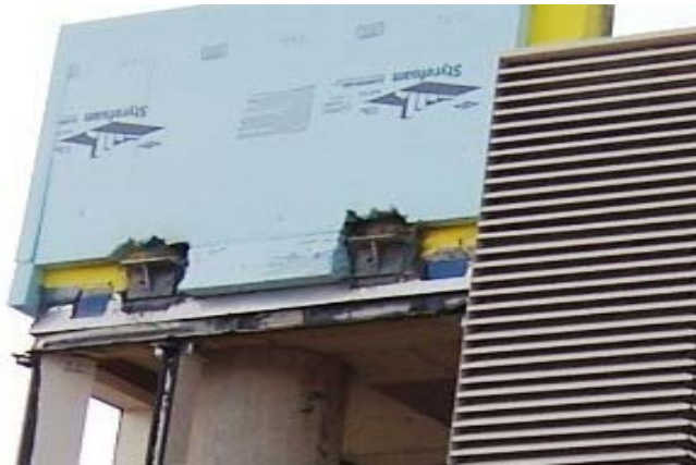
Figure 3: Mock ups help determine contractor sequencing and discover potential issues prior to actual installations on the building
