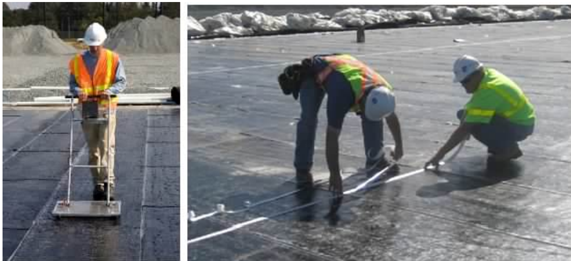
Figure 6. Survey followed by leak locate grid installation on a large reservoir membrane
