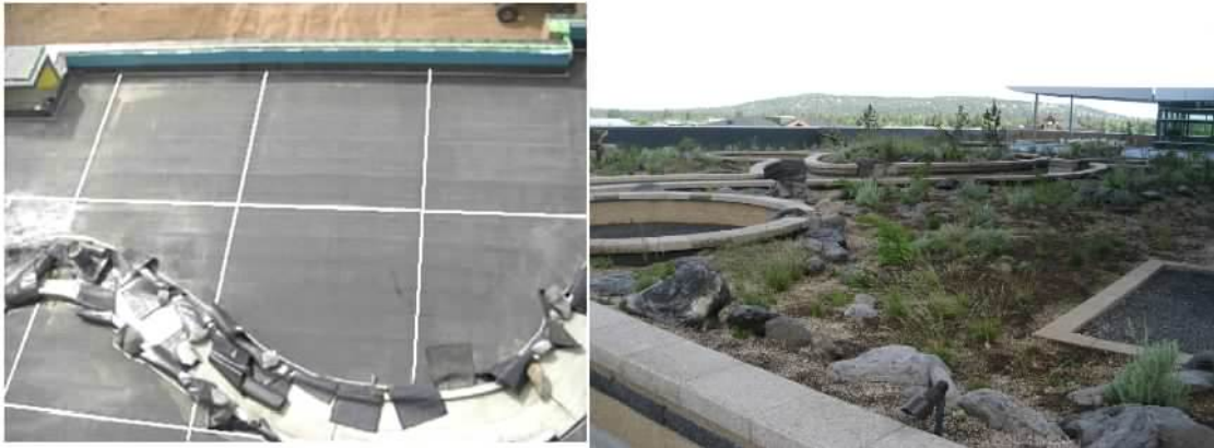
Figure 5. Leak locate grid installed on membrane of an intensive green roof system
