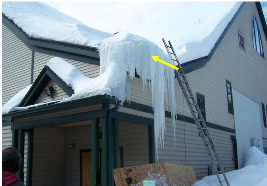
Photo 1 – Severe icicle and ice dam formation at metal roof eave.
