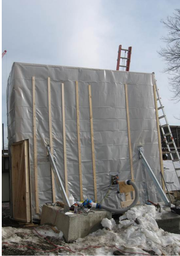
Photo 5 – Air leakage testing of construction mockup of an exterior wall assembly with a fenestration.
