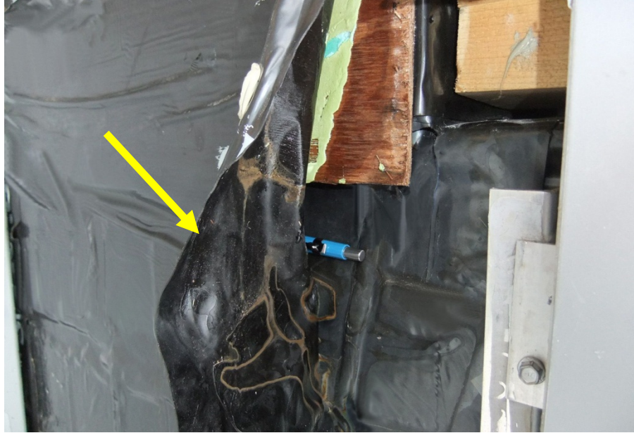
Photo 7 – Membrane edge (arrow) of air barrier sheet is not adhered to sheet of adjacent air barrier assembly.
