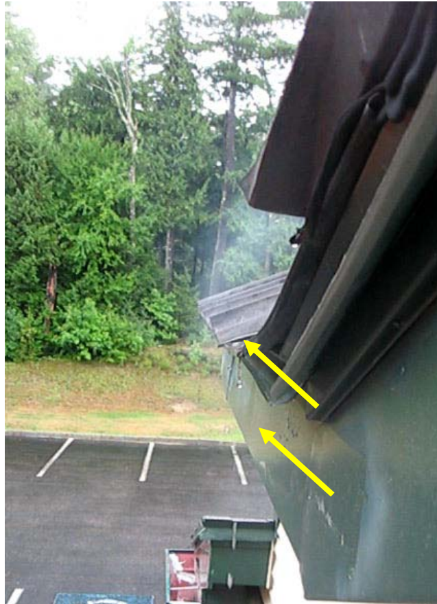
Photo 10 – Tracer smoke exfiltration at roof eave (arrow).
