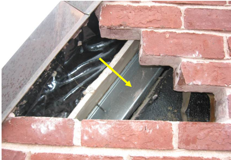
Photo 4 – Discontinuity in air barrier system at roof-to-wall intersection. Note the exposed metal roof deck and lack of integration between roof air barrier membrane and fluid-applied wall air barrier (arrow).
