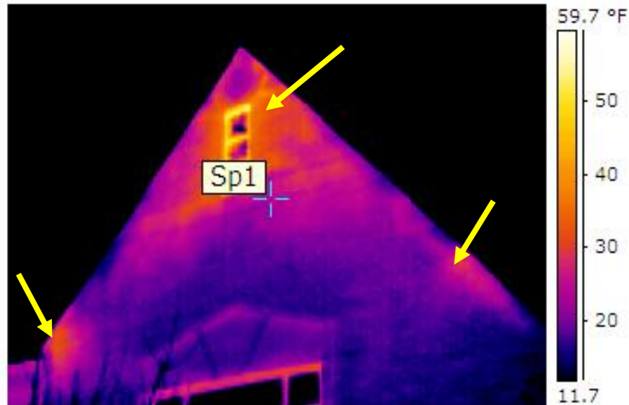
Photo 11 – Infrared image of exterior wall taken during the winter in a heating climate. Orange/yellow regions indicate locations of elevated heat loss (arrows).
