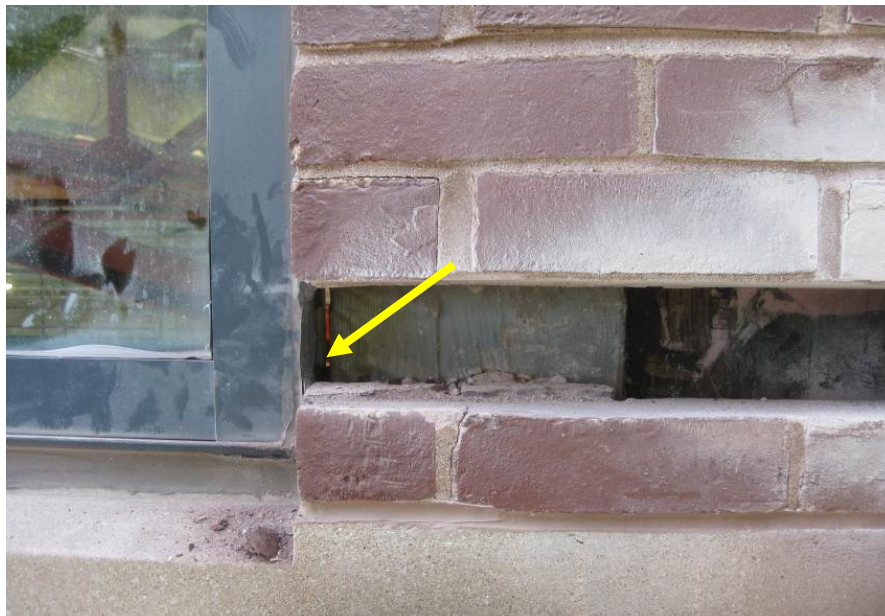
Photo 3 – Air barrier discontinuity at window-to-wall air barrier transition (arrow illustrates unsealed gap to building interior).
