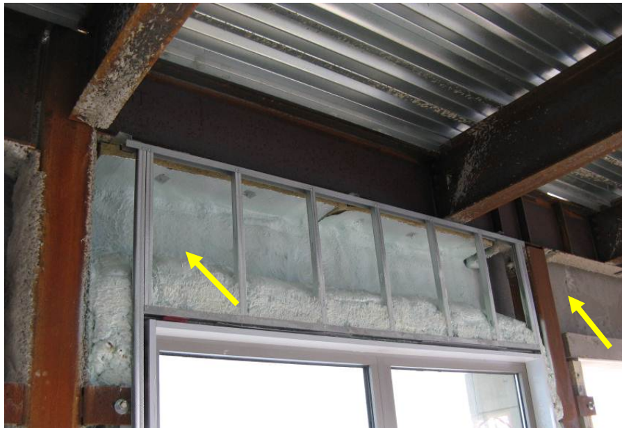
Photo 2 – SPuF insulation applied to inboard side of precast concrete wall panel (left arrow). Right arrow illustrates precast concrete panel.
