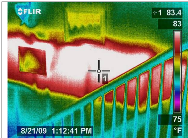
Figure 2 Infrared image at stairwell shows that floor space behind wall is very warm. (Image credit C. Withers)
