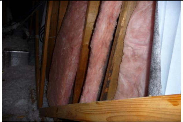
Figure 6 Insulation batts are not consistently in close contact with the wallboard, allowing considerable convective heat exchange between attic air and wallboard, as shown in Figure 4. (Withers)
