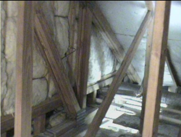
Figure 7 Photo of IR image above. The floor cavity at the bottom of the wall is open to garage attic. (Withers)
