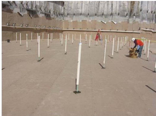
Image 2 – Bentonite waterproofing membrane installed over rat slab and sealed around tie-down penetrations
