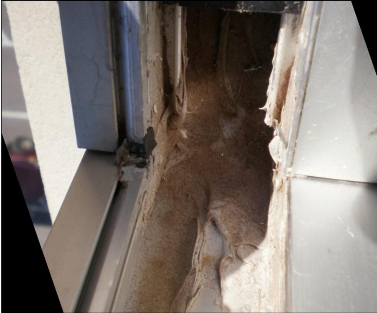
Figure 4: This is a typical end dam condition at a horizontal-to-vertical window mullion intersection. Checking window end dams by blocking the weep holes and filling the horizontal with prior to glass installation will save the Building Owner from future problems and costs.
