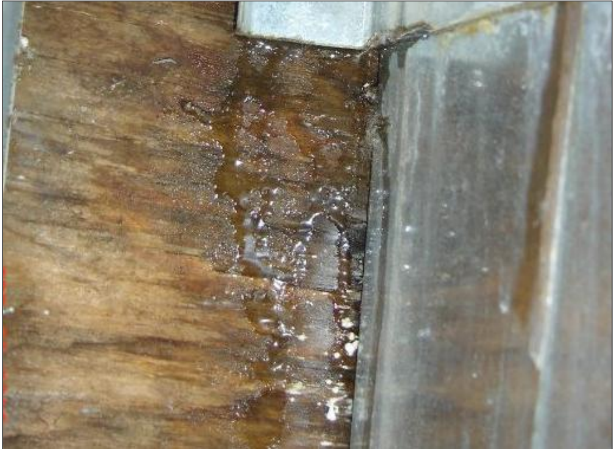
Figure 7: Water penetration in the wall cavity can go unnoticed if not evident from the interior of the building. This can eventually lead to hidden organic growth.
