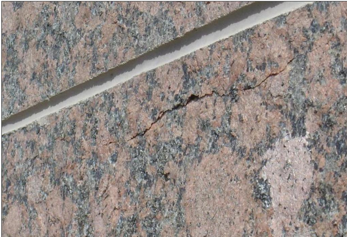
Figure 2: Cracks in Veneer cannot only allow water penetration, but can be a sign of structural instability in the cladding.
