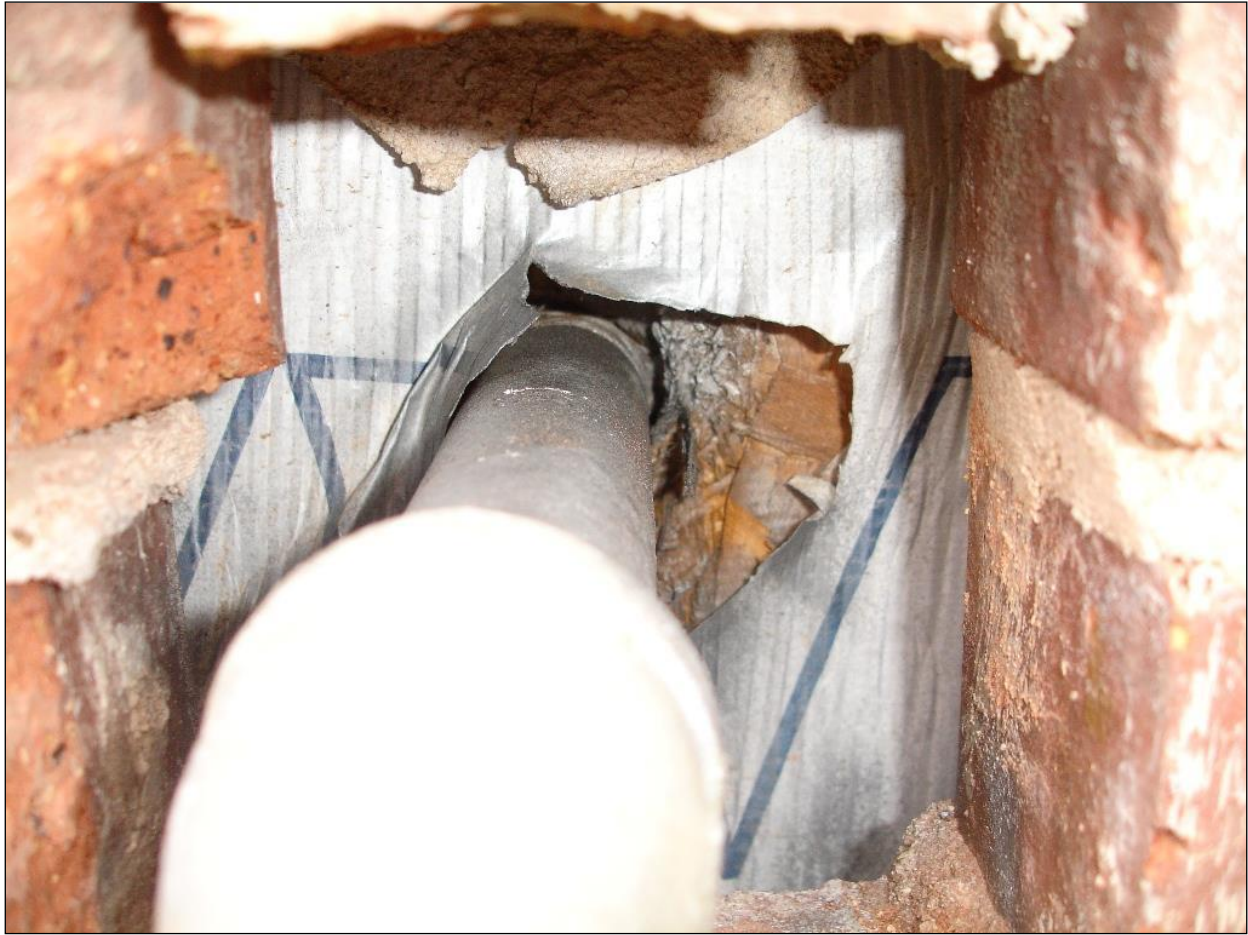
Figure 5: Hidden breaches and installation defects in the water-resistive barrier can allow water into the wall cavity and building interior.
