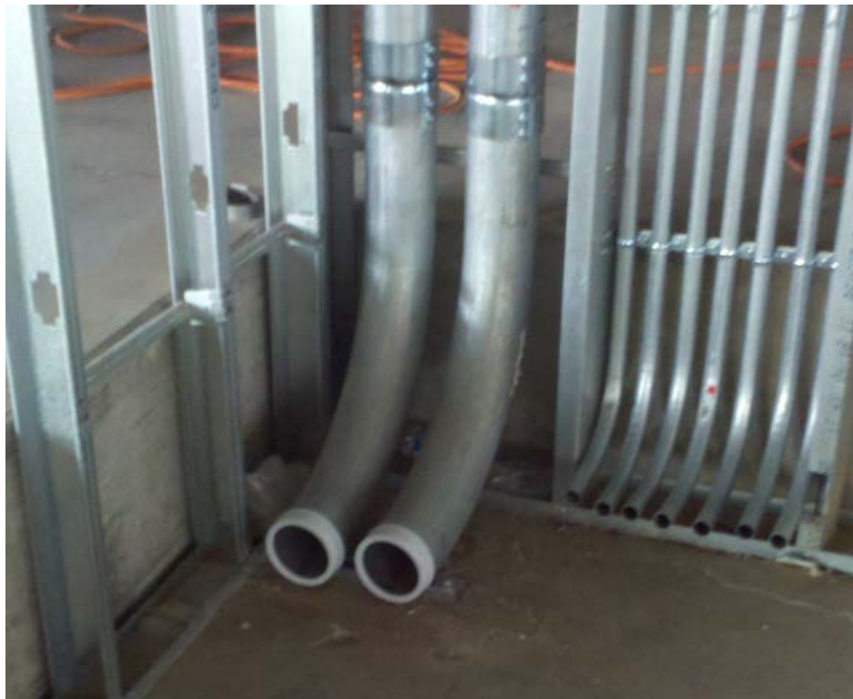
Figure 5 - Open Ended Conduits within the Access Floor Plenum
