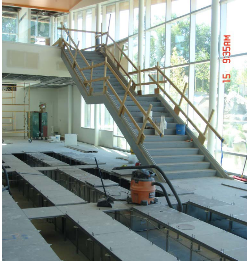
Figure 1 - Typical Office Access Floor (lobby installation shown)
