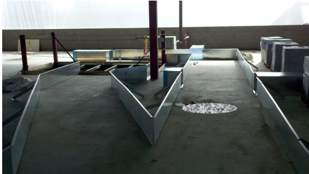
Figure 3 - Air Highway Prior to Access Floor Installation (note vertical chase opening in background)
